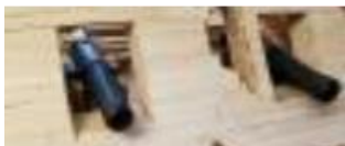
View of casement anchor chain pipes. Pipe on left is cut to 45 degrees to match face of casement. Pipe to right is actually for the inside of casement wall and flared to allow chain movement to capstan. These will be glued in place after armor is applied to front of casement and casement is permanently attached.
